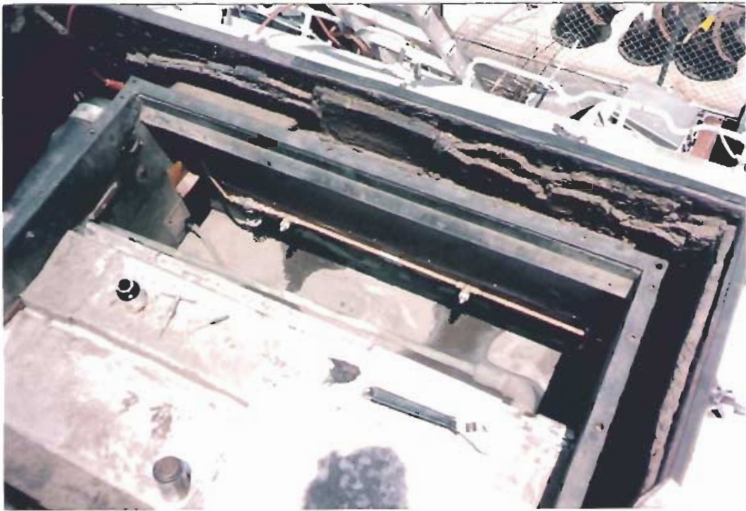
FIG 23 AC CONDENSER UNIT
